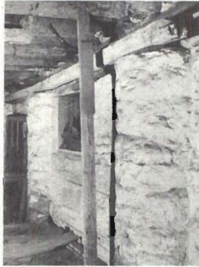
One corner of J. B. Vallé basement is occupied by room with massive stone walls, believed to be foundation for old fort.
