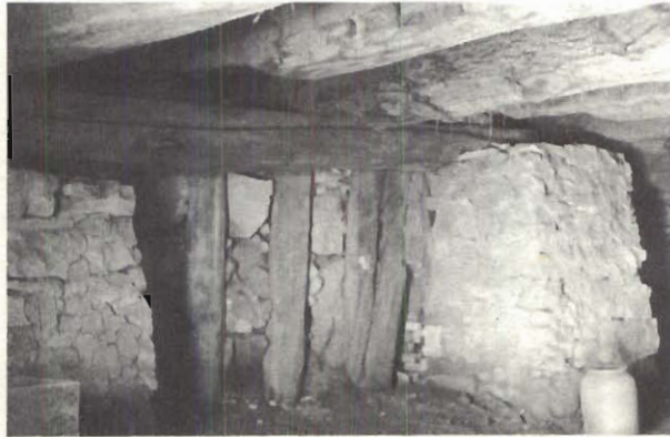
Great oak beams are reinforced by rubble stone buttresses in Amoureux foundation.
