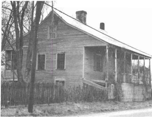
Excellent old Ribault house still is sturdy despite years of neglect.
