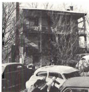
Old two-story LaBruyere home now is occupied by junk dealer. Note how porches are sinking from core of house.
